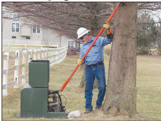
Cuivre River Electric Cooperative Crew Chief Craig Larkin demonstrates pad-mount transformer accessibility challenges that line workers face daily. Workers need at least 10 feet of clear space in front of pad-mount transformers to maintain a safe working distance. The fiberglass hotstick is designed to provide about 10 feet of "elbow room" in front of the access panel. Cuivre River Right-of-Way personnel worked with the property owner at this site and the tree has since been removed to allow proper transformer access.
