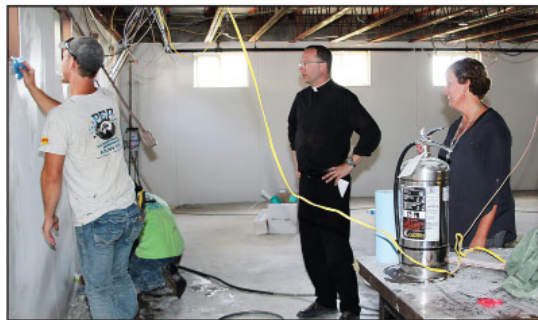
Father Jason Duke and Lori Schuckenbrock, principal at St. Clement School, check on work being done in the school's basement. Rain and mold forced the parish to completely renovate. The parish is holding an auction on Sept. 16 to raise money to help with expenses.
