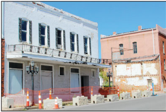
The building known as the old gas company is located at 16 S. Court Street and shares a wall with MASH. It is owned by William Butler and Conita Butler. It's also behind the other dangerous property at the corner of Main and Court Streets owned by Gary Rahmeyer. Both structures have been deemed unsafe and will have to be demolished before the street can reopen to traffic. The street was shut down following an engineer's inspection on Monday, Sept. 11.
