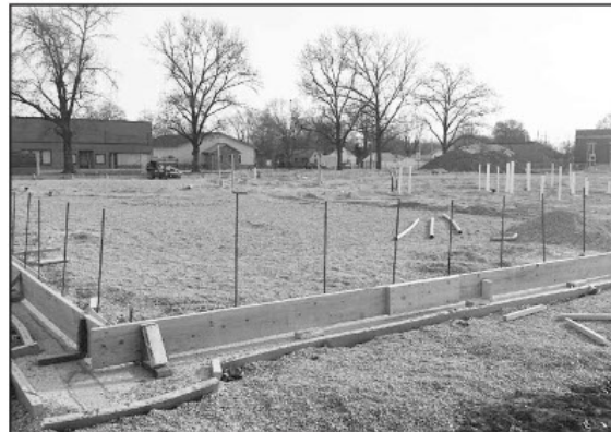
Pictured is the Eastern Missouri YMCA plumbing and electrical groundwork at the site on Main Street in Vandalia.
