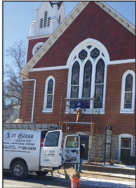
Art Glass Unlimited of St. Louis erects scaffolding Jan. 18 along the east-facing stained glass window at Clarksville United Methodist Church.
