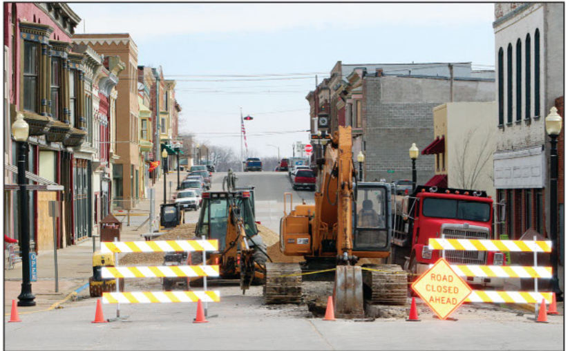
Work has officially started on the Georgia Street corridor project. Funding for the project was squared away in February and aspects of the enormous project were put out for bid. It has taken two years of meticulous planning to set up the $4,000,000 endeavor that was sorely needed. The project will include replacing old infrastructure with new water distribution and wastewater lines as well as addressing storm water collection, streets and sidewalks. Motorists are urged to use caution and to be patient during construction.
