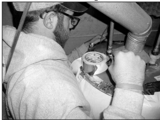
NECAC's Hunter Northcutt installs a new hot water heater as part of the agency's weatherization efforts. NECAC made improvements to more than 400 homes as part of home ownership and housing development projects in the last 18 months.
