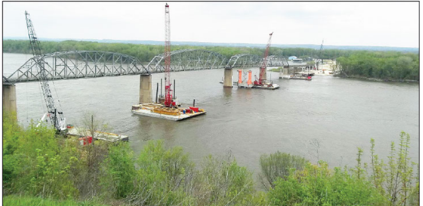
A view of the Champ Clark Bridge on May 2, 2018, with construction of the new bridge taking place. (Courtesy Brent Engel)
