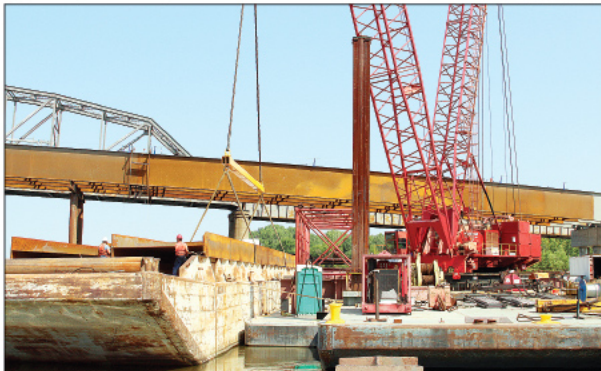
Crews prepare one of the steel girders to be lifted by crane and placed along the piers. Construction of the new bridge is about the halfway point and is projected to be open to traffic by November of 2019. Trib photo by April M. Frorick
