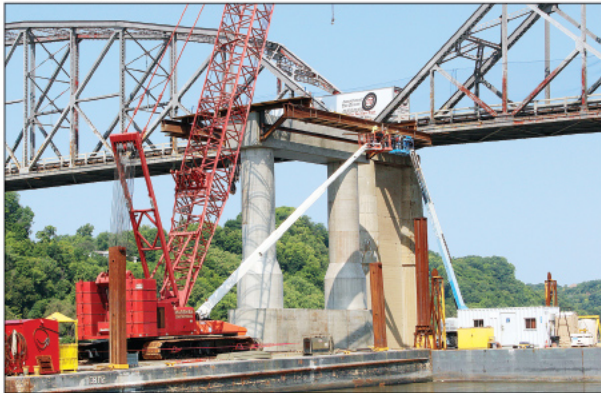
On Friday, Aug. 3, crews were working to prepare one of the steel-reinforced concrete piers for the steel girders that will be placed on it prior to the decking. Trib photo by April M. Frorick
