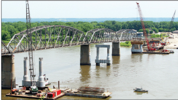
Work has progressed over the past year and has become more visible lately as crews have worked to drill through 24-feet of bedrock to place the steel-reinforced shafts for the concrete piers that will hold the steel girders and concrete bridge deck. The photo above was taken earlier this year. Trib photo by April M. Frorick
