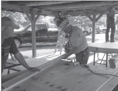
Rotary members work on installing new boards for the ceiling, from left: Wendel Tabert, Tim Embree (on ladder), Rennie Davis and J.C. Davis
