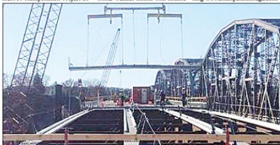
Work is already past the halfway point on the new Champ Clark Bridge in Louisiana. Over the next few months the majority of work will be focused on the placement of the remaining deck panels and completing closure joists between panels.
