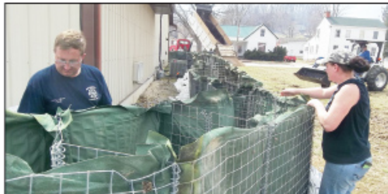
Larry LaFave of Eolia and Jessica Witt of Louisiana put a berm in place March 24 around American Legion Post 349 in Clarksville as more sand is delivered by a dump truck. The berm was to be filled with sand.
