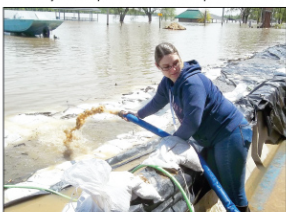
Kristen Boyette of the not-for-profit North East Community Action Corporation (NECAC) pumps deep water from the area in front of the Clarkville Apartments.
