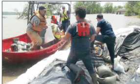
Volunteers unload sandbags Sunday to reinforce a makeshift flood levee at the corner of First and Washington in Clarksville. Delivery by boat where vehicles once traveled is the quickest method of getting bags where they're needed the most.
