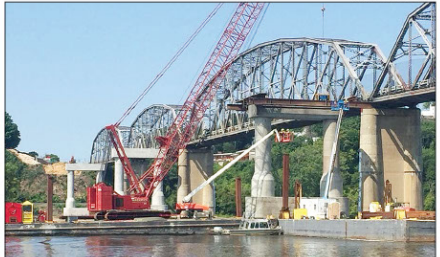
Construction of the new Champ Clark Bridge reached the halfway point in late July of 2018. Trib photo by April M. Frosio
