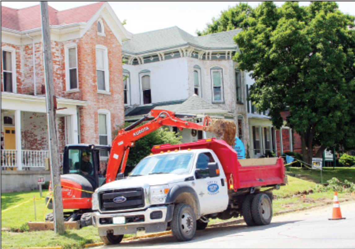
City crews have been working throughout the summer on the Georgia Street project. The street will have new water distribution lines, storm water drainage and sanitary sewer lines, along with new pavement and new sidewalks on the south side of the street. The city is also working with various utility providers to replace lines before work is completed to ensure work doesn't have to be disturbed once done. The city has been working on the sanitary sewers and water mains along with utilities. New pavement, curbs and sidewalks should be completed by next summer.
